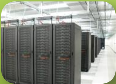
Datacenter Colocation Generation 1
